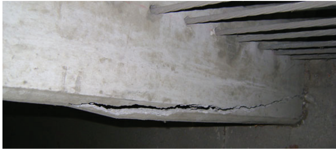
Cracking due to poor structural design
