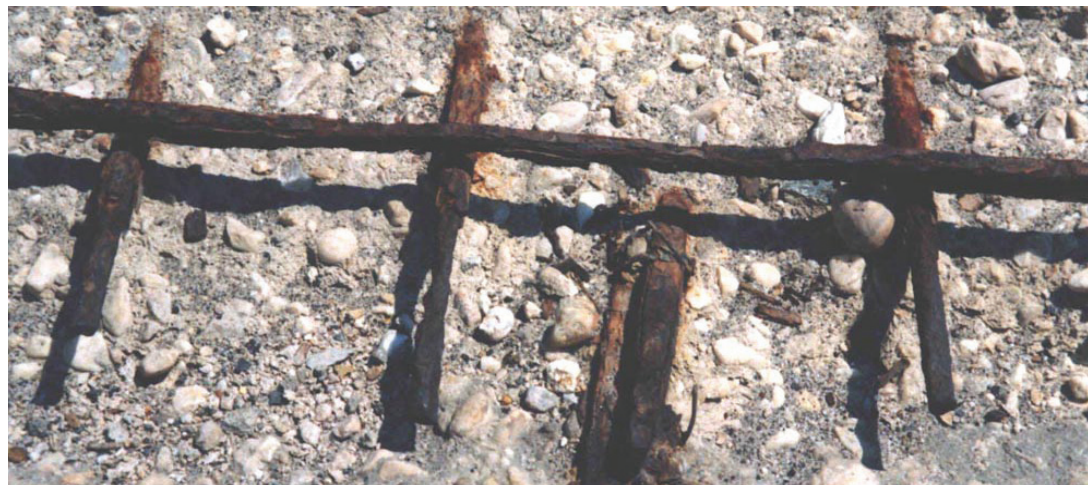
Chloride corroded reinforcing steel
